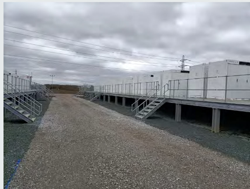
Pillswood Battery Storage site near Hull, operated by Harmony Energy Income Trust
